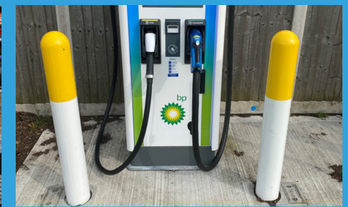
A barrier around a public rapid chargepoint
